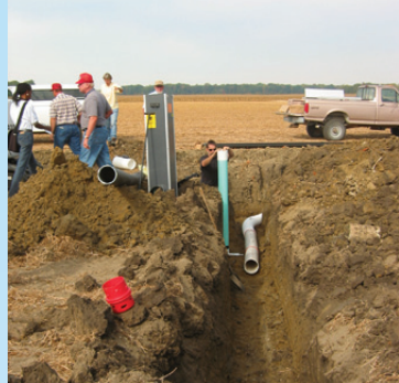
Drainage monitoring installation, DPAC Site, IN
