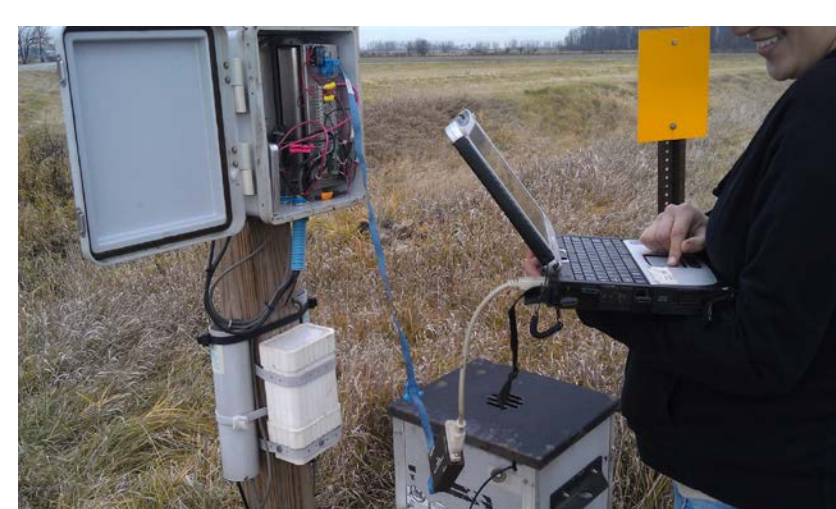
Water levels inside the control structure were downloaded to calculate flow rate
