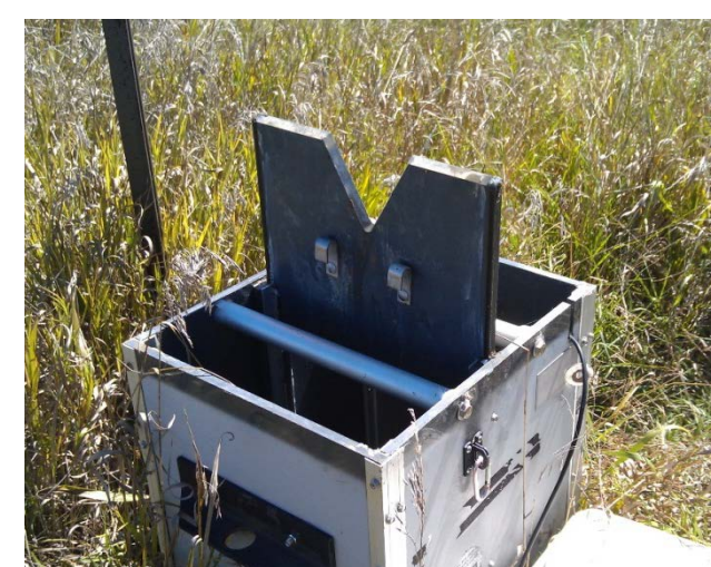
V-notch weirs were placed in each structure to improve the accuracy of the flow rate calculation at low flows
